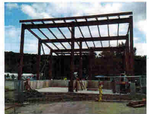
Workers construct the metal frame of the food scraps transfer building at the Recycling and Solid Waste Center in late September.
